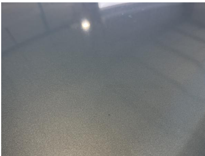
5: Roof Scratched Over 25mm Thru Paint
