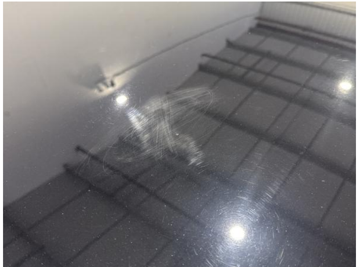
12: Roof Scratched Over 25mm Thru Paint
