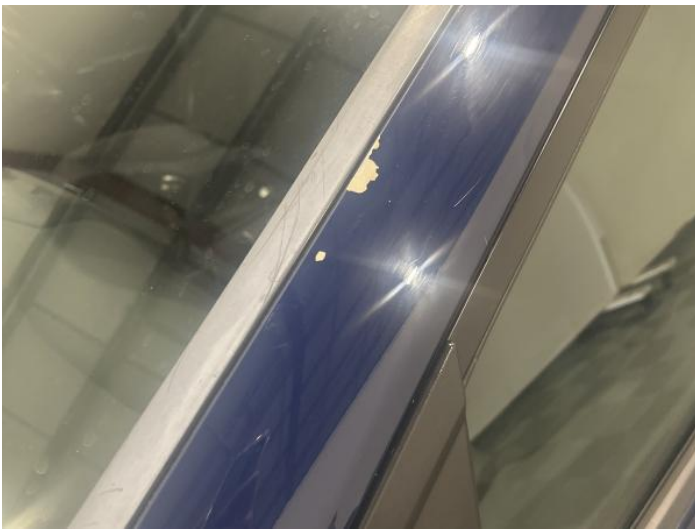
23: A Post ns Poor Previous Repair Paint Flake
