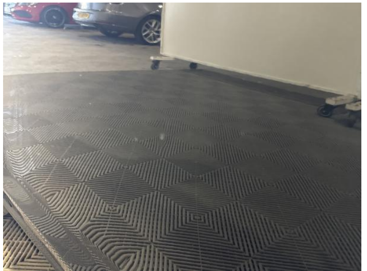
6: Door nsf Chipped 1 To 5
