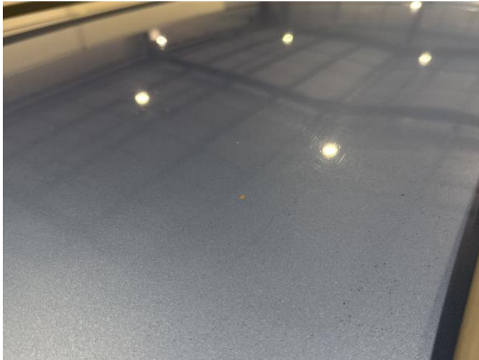
21: Roof Dented Over 30mm
