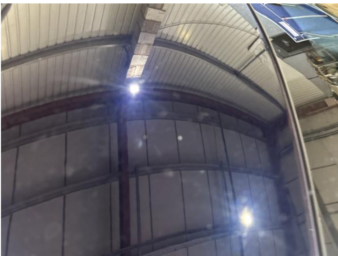
13: Roof Chipped 1 To 5
