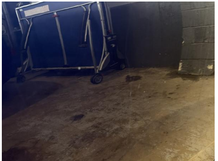
2: Door osf Chipped 1 To 5
