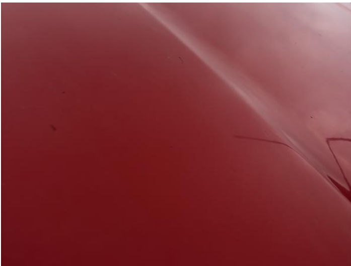
17: Roof Dented Over 30mm
