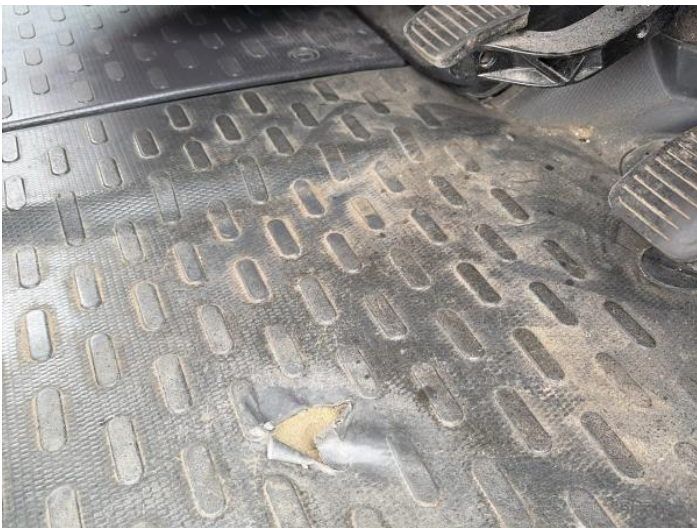
1: Carpets Front Broken Replace
