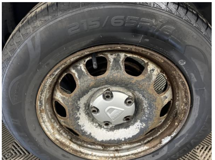
14: Wheel nsr Corroded Light
