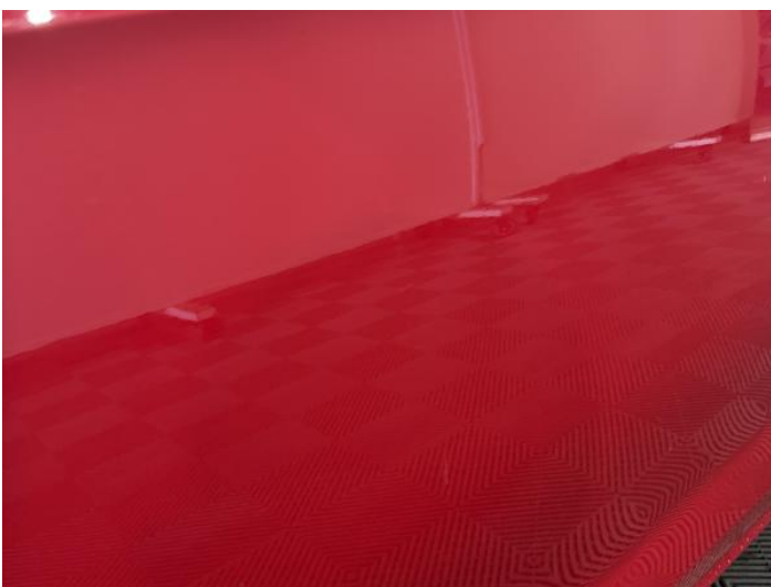
7: Door nsf Scratched Over 25mm Thru Paint
