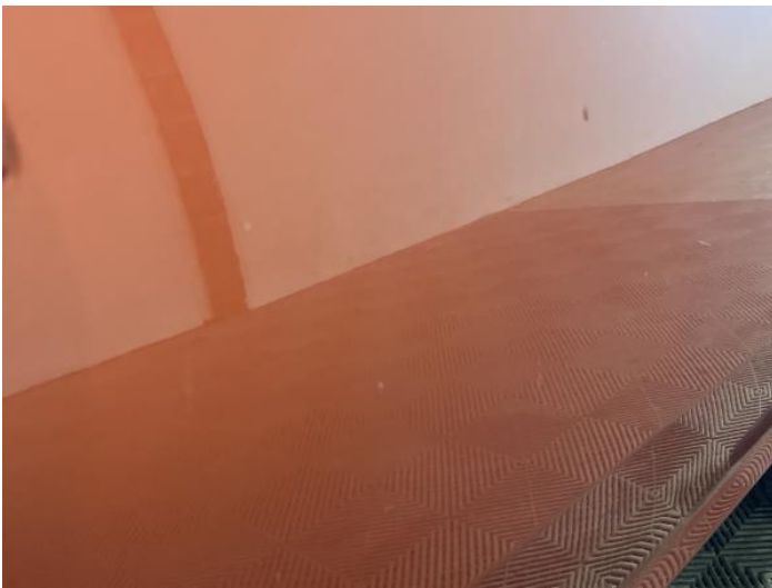
11: Door osf Scratched UpTo 25mm Thru Paint
