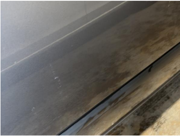
5: Door nsf Scratched Over 25mm Thru Paint
