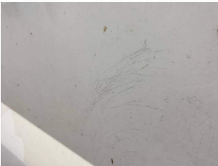
13: Door nsf Dented With Paint Damage
