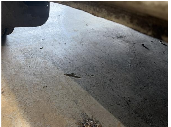
12: Sill ns Scratched Rusted
