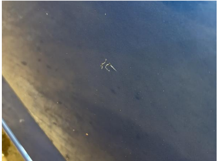
16: Door nsf Scratched UpTo 25mm Thru Paint
