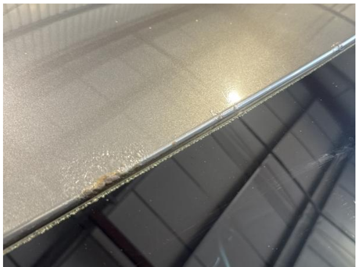
20: Roof Rusted Over 5mm
