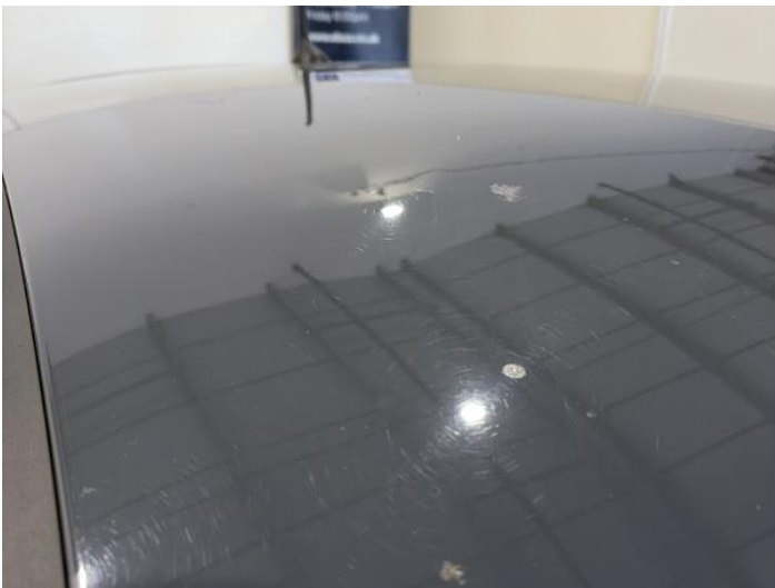
17: Roof Dented Over 30mm
