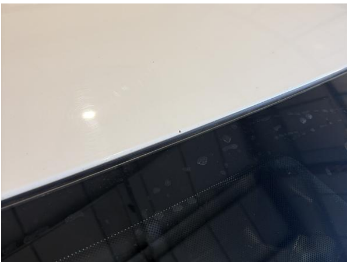
13: Roof Chipped 1 To 5
