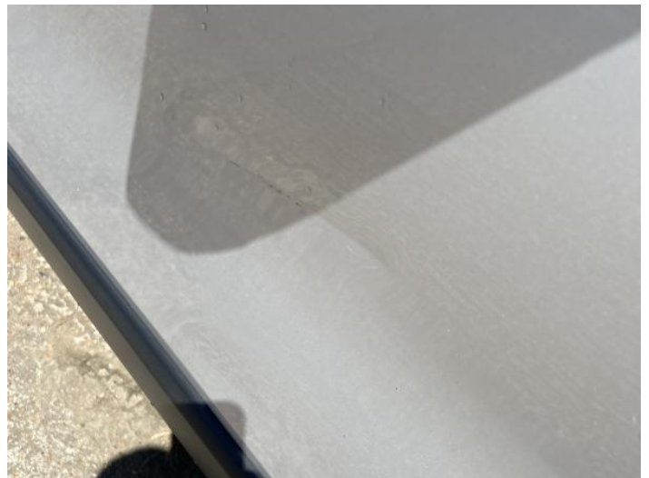
2: Door of Dented With Paint Damage
