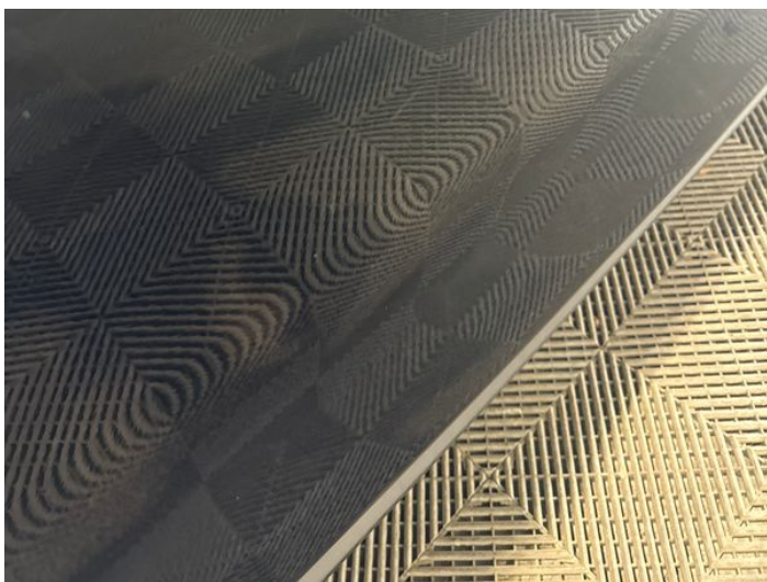
17: Door osf Scratched UpTo 25mm Thru Paint
