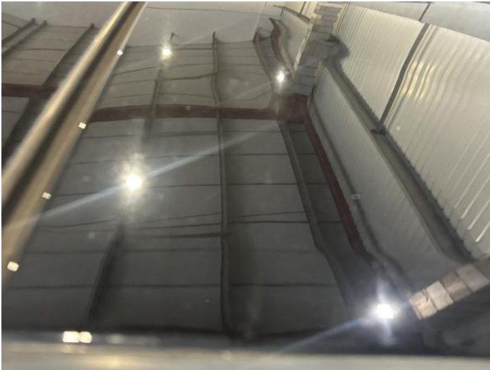
21: Roof Dented Over 30mm
