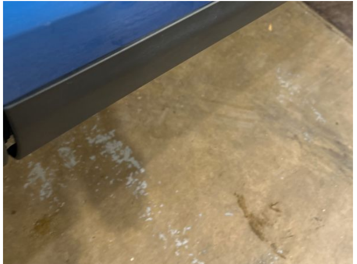
4: Door osf Dented Between 10mm + 30mm
