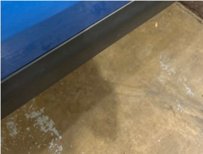
3: Door osf Chipped 1 To 5
