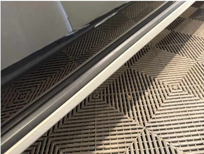
5: Door nsf Scratched Over 25mm Thru Paint
