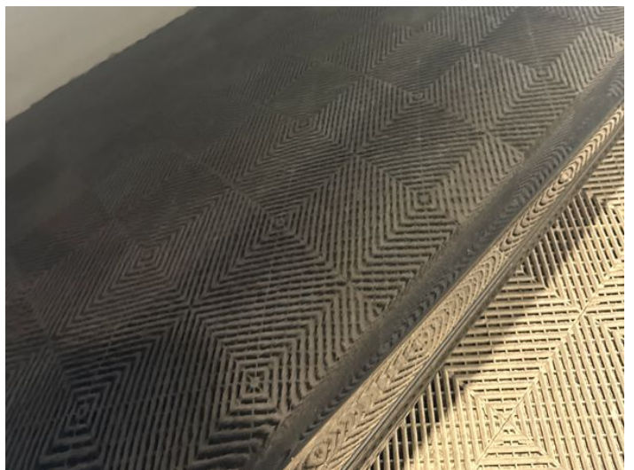
14: Door osr Scratched UpTo 25mm Thru Paint
