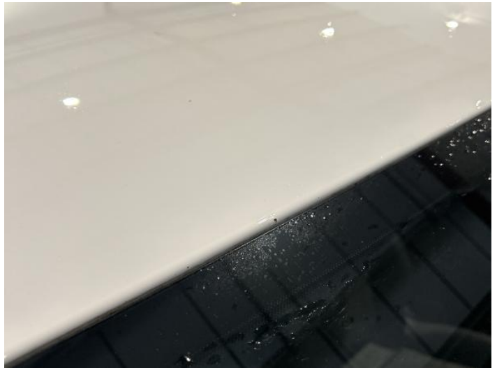
12: Roof Chipped 1 To 5
