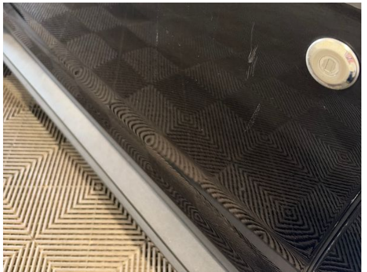
6: Door nsf Scratched Over 25mm Thru Paint
