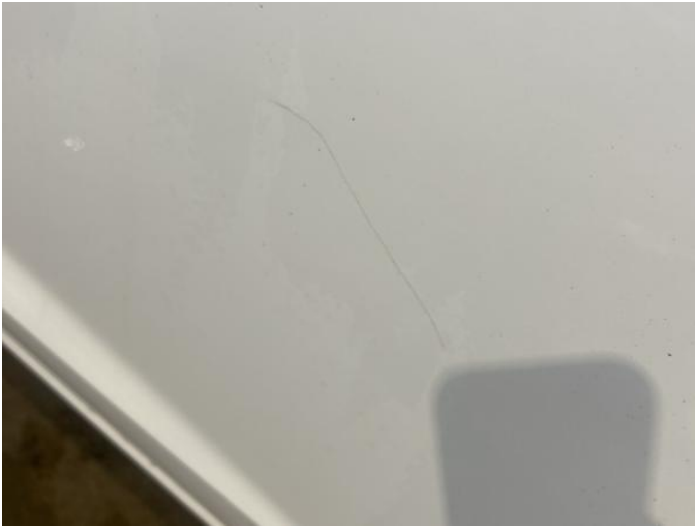
3: Door osf Scratched Over 25mm Thru Paint
