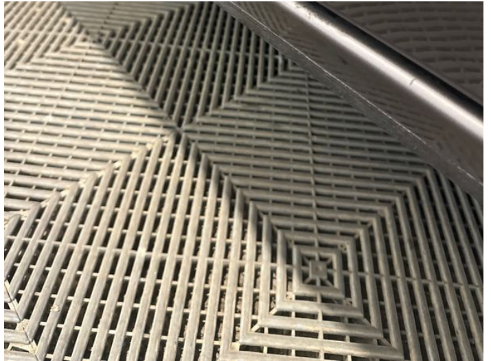
16: Sill os Scratched Over 25mm Thru Paint
