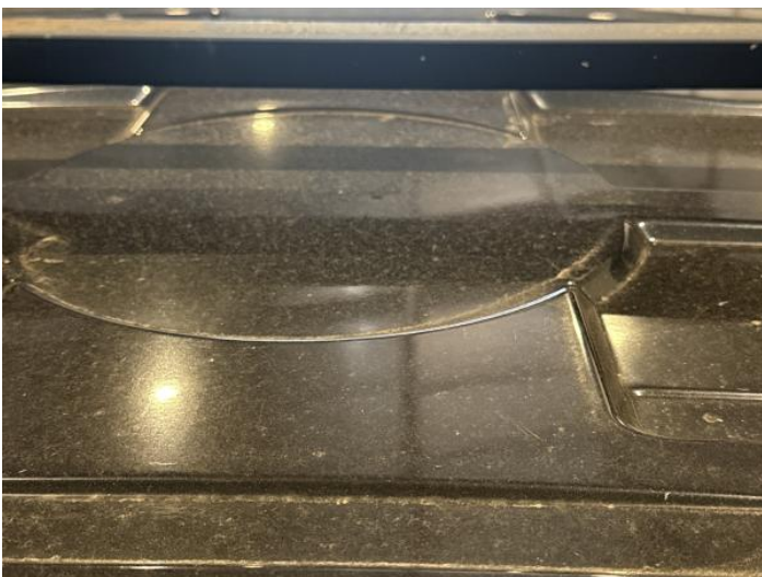
19: Roof Dented Over 30mm
