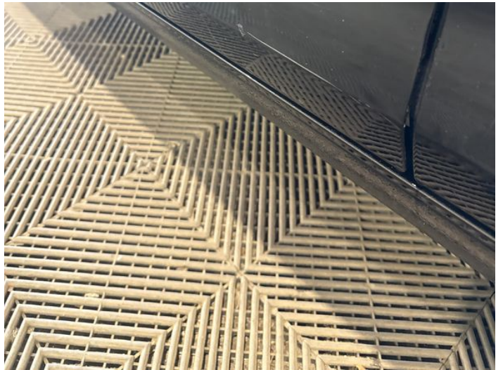
6: Door nsf Scratched Over 25mm Thru Paint
