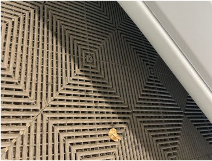
3: Sill os Rusted Over 5mm
