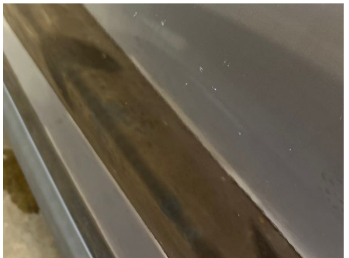
8: Door nsf Chipped Multiple Chips
