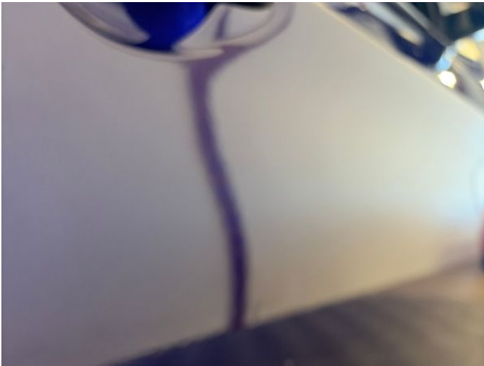
17: Door osf Dented Between 10mm + 30mm
