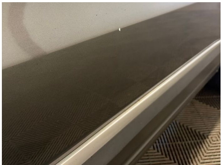
20: Door osf Chipped Edge Chip
