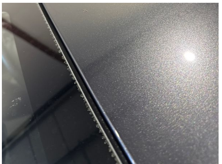
20: Roof Rusted UpTo 5mm
