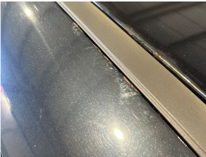
11: D Post ns Rusted Over 5mm
