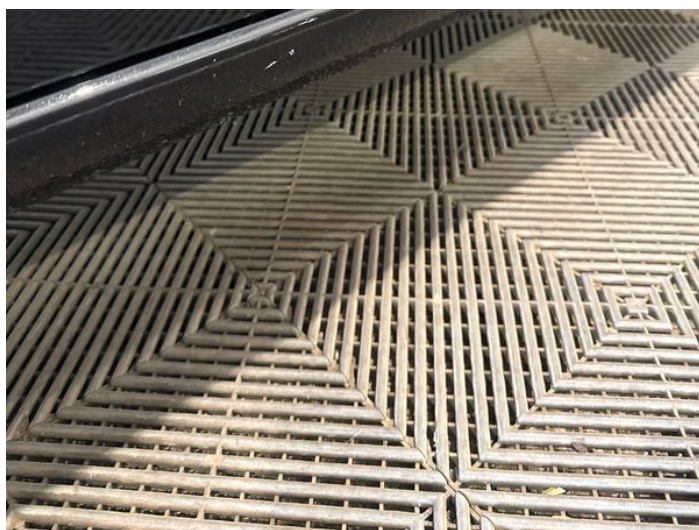
8: Sill ns Scratched UpTo 25mm Thru Paint
