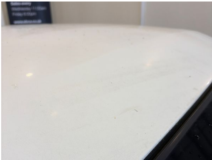
21: Roof Chipped 1 To 5
