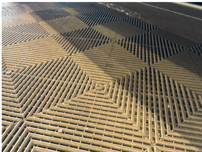
10: Sill ns Dented With Paint Damage
