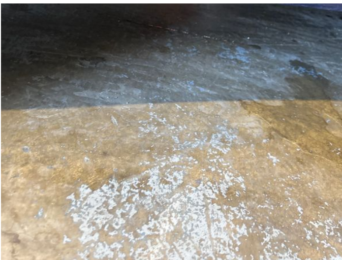
19: Sill os Rusted Over 5mm
