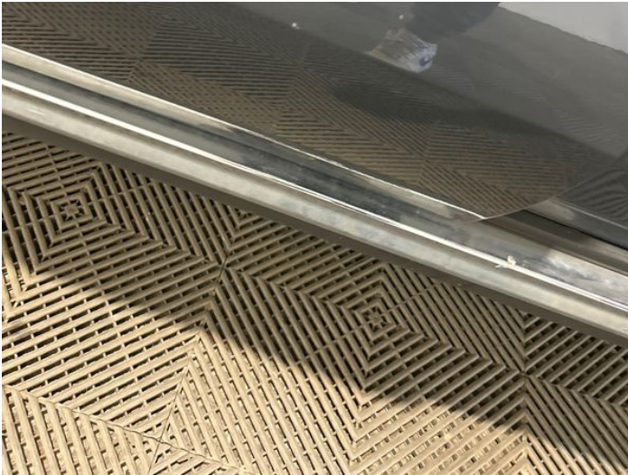
3: Door osr Chipped 1 To 5
