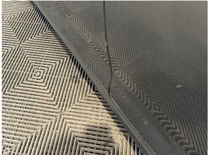
16: Door nsf Chipped Edge Chip
