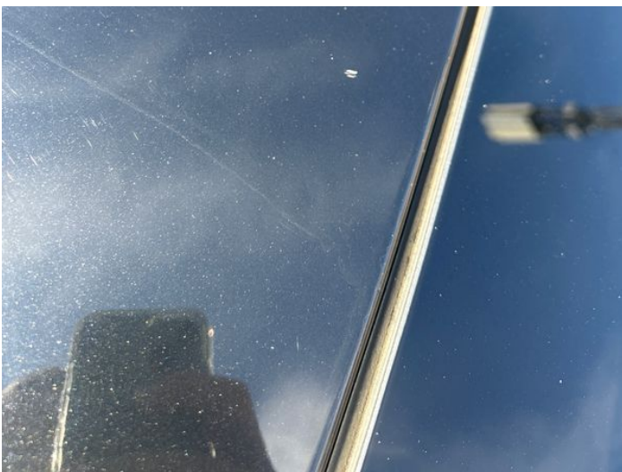
19: Roof Chipped 1 To 5
