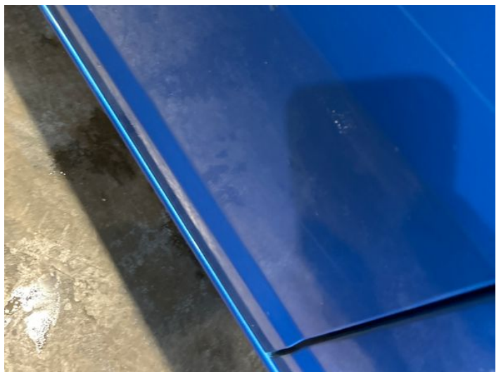
14: Door nsf Chipped 1 To 5
