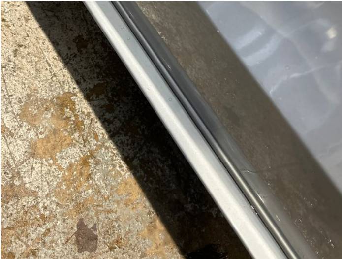
3: Door osf Chipped 1 To 5
