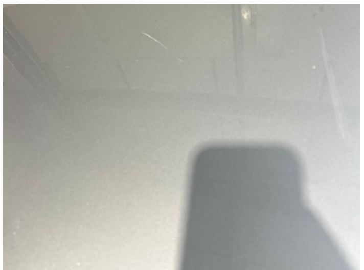
20: Roof Scratched Over 25mm Thru Paint
