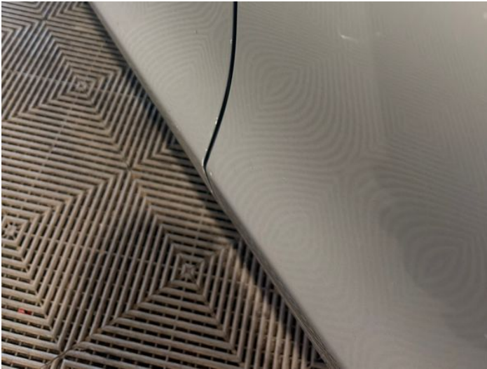
15: Door nsf Chipped Edge Chip
