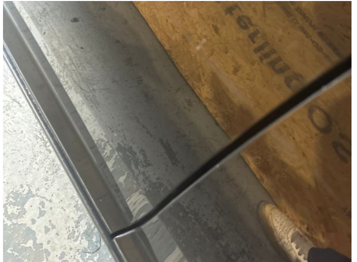
10: Door nsf Chipped 1 To 5
