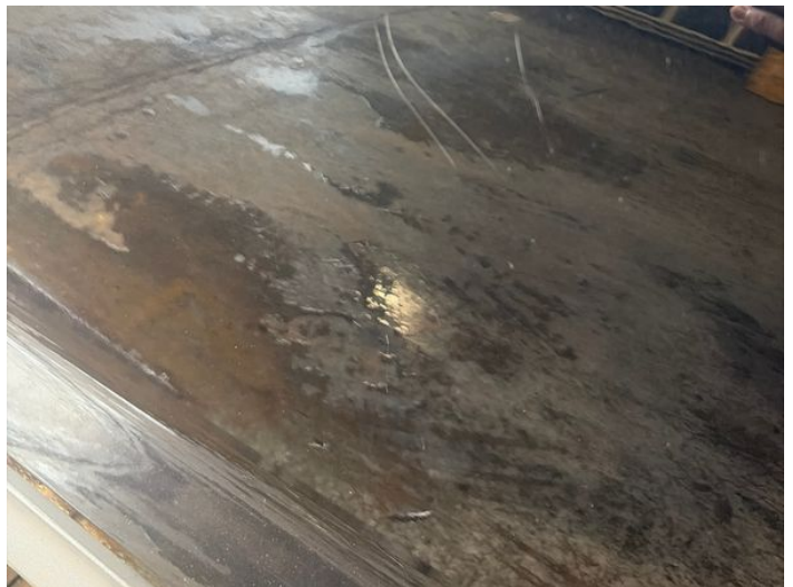
12: Door nsf Scratched Over 25mm Thru Paint
