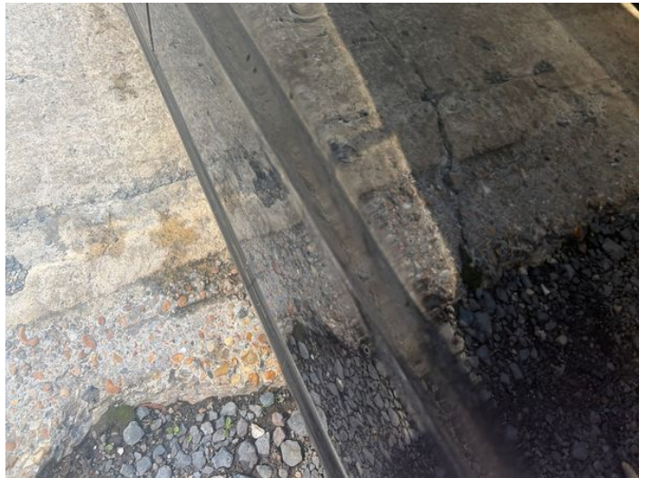
12: Door nsr Dented Between 10mm + 30mm
