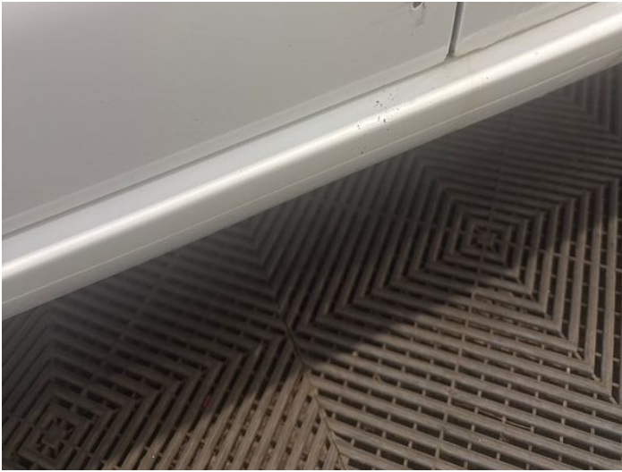
9: Door nsf Chipped Over 5mm
