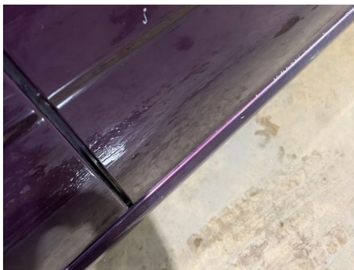
2: Door osf Scratched UpTo 25mm Thru Paint
